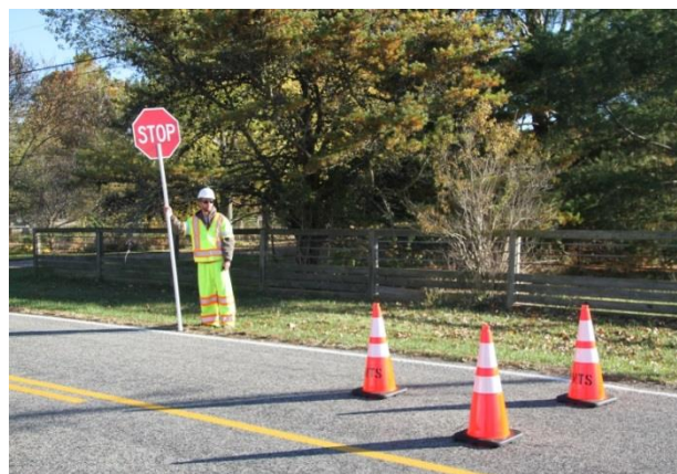
An example of new Class 3 reflective wear requirement for flaggers and placement of three cones 15 feet in front of the flagger position.
